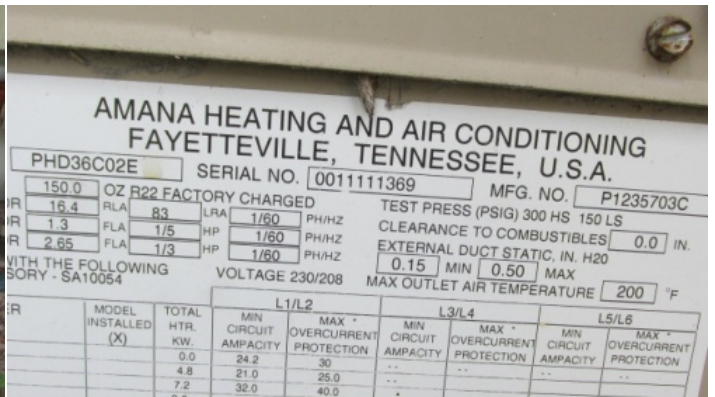
Heating & AC package unit label - mfg 2000
