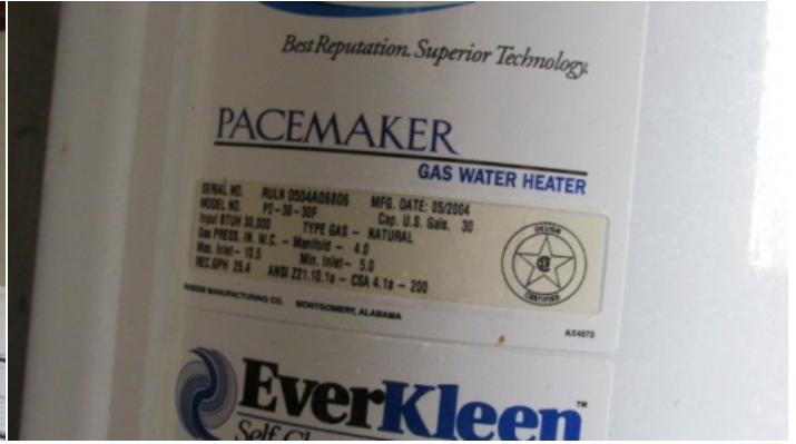
Water Heater label - mfg 2004
