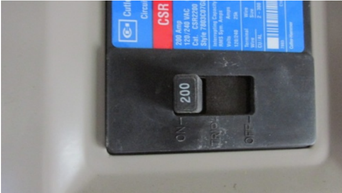
Main Breaker - 200a
