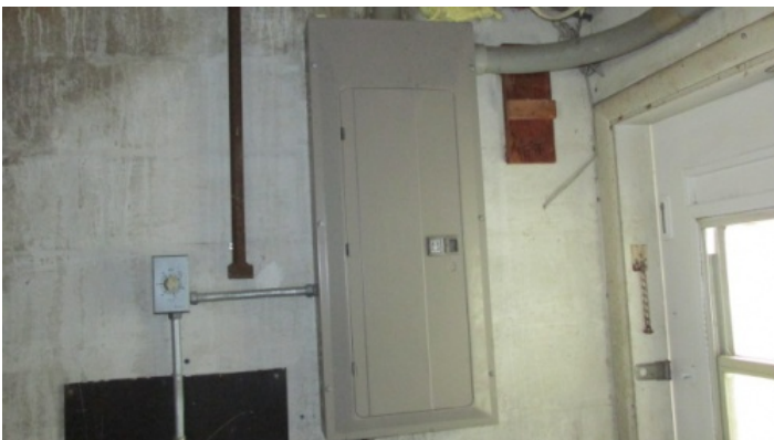
Electrical Distribution Panel (cover on)
