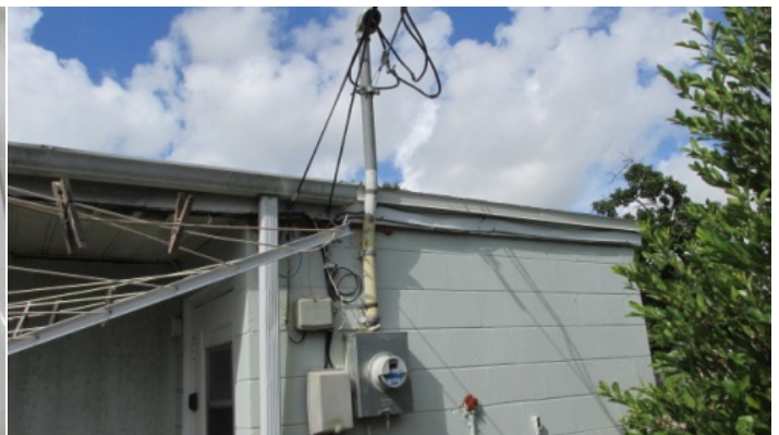
Electrical Service to Home (at meter)
