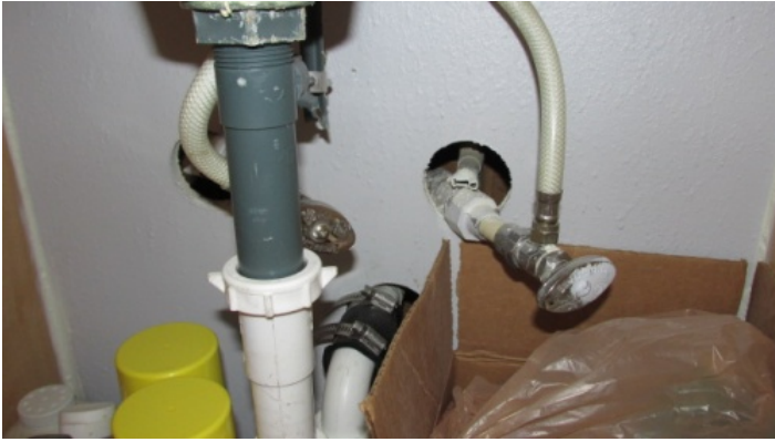
Bath Plumbing (under sink) - shut off valves, flex vinyl water supply lines
