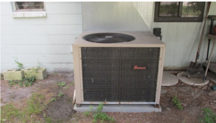
Heating & AC package unit
