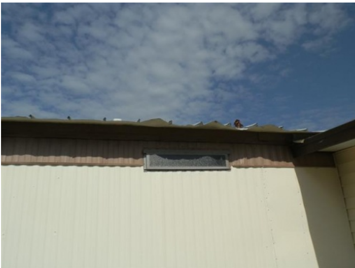
Roof Damage Observed
