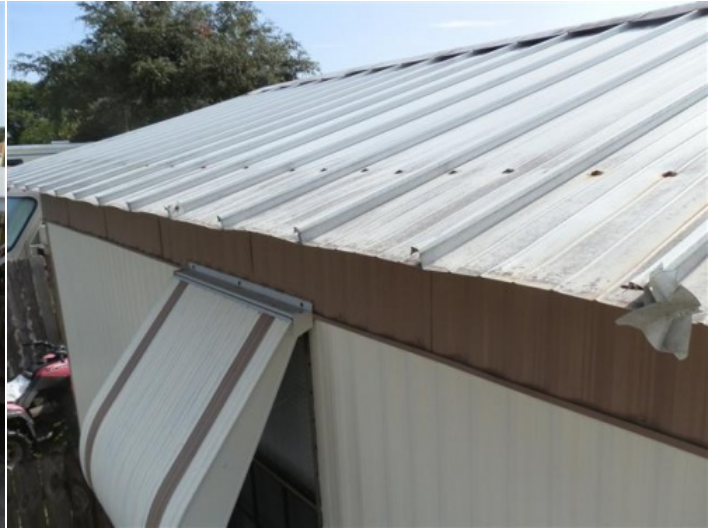
Metal Fascia Has Been Removed
