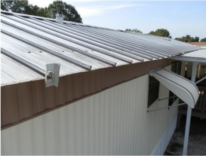
Metal Fascia Has Been Removed
